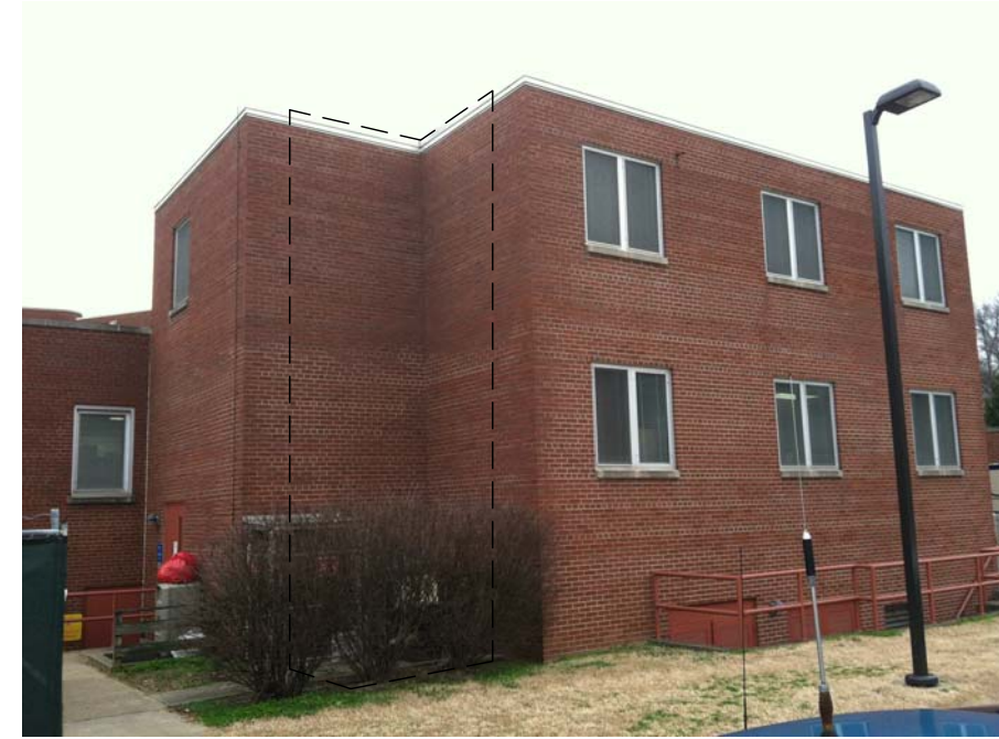
SITE OF NEW ELEVATOR REF.: DEMOLITION NOTES D.11 THROUGH D.14 AND 1/D010, 2/D010, AND 3/D010
