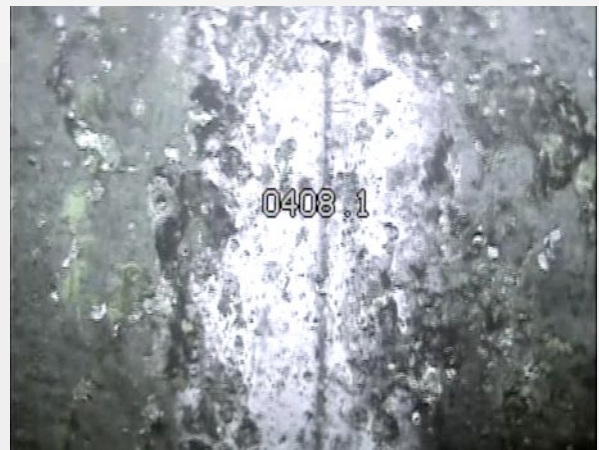
Vertical Casing Seam
