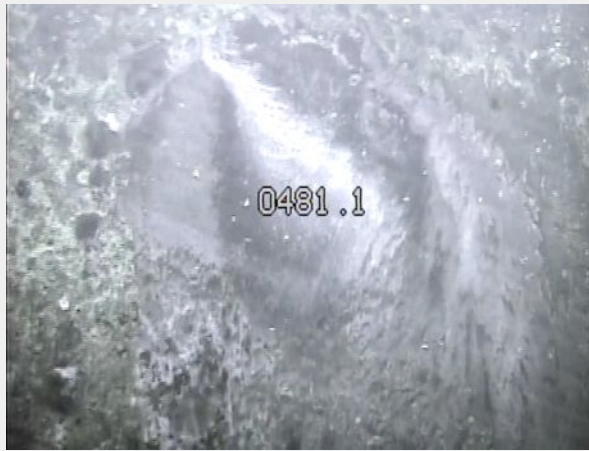
Scour Marks caused by the pump
