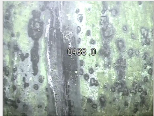
Vertical Casing Seam
