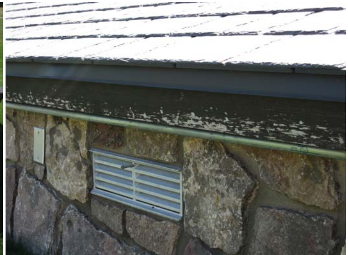
Figure 8: Shelter fascia board (typical) to be stripped and repainted
