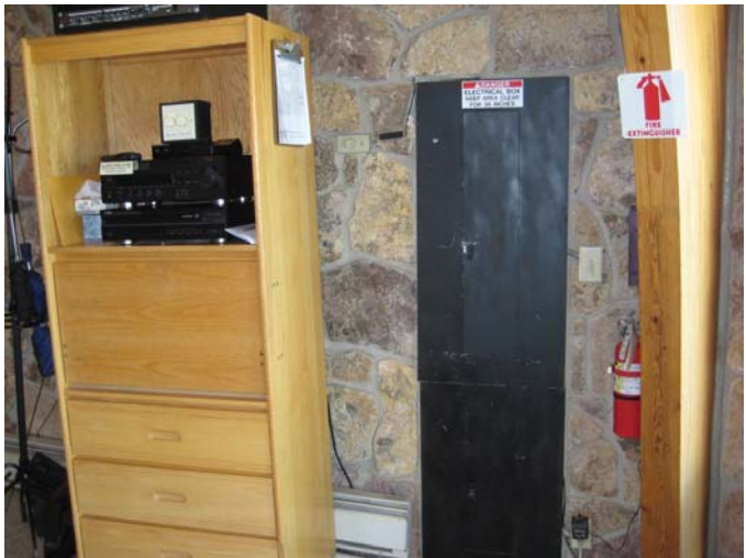
Figure 2: Shelter interior electric panel (top C/B enclosure) to be removed and replaced
