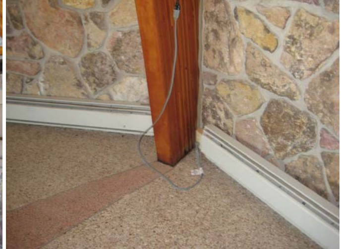
Figure 6: Shelter electric baseboard heater (one of two) with receptacle to be replaced with factory installed type
