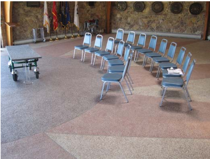
Figure 1: Shelter “rustic” terrazzo floor to be refinished
