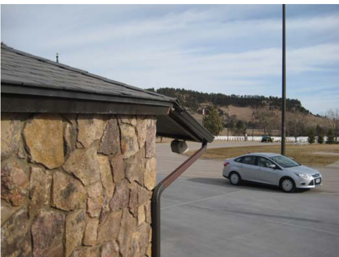
Figure 9: Shelter downspout, end of run
