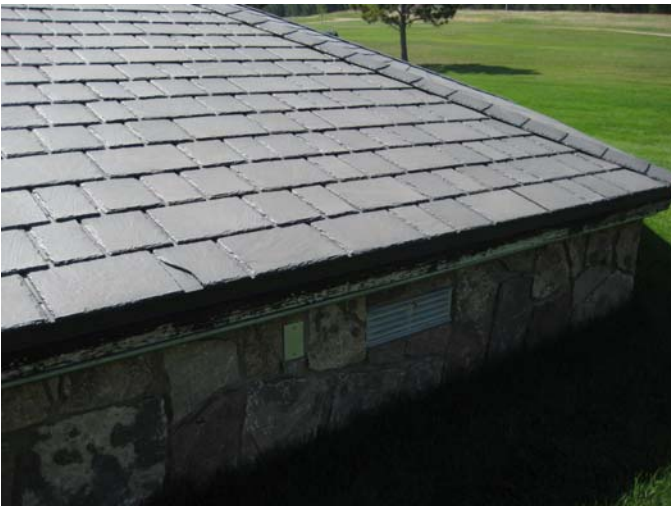
Figure 7: Shelter fascia board (typical) to be stripped and repainted
