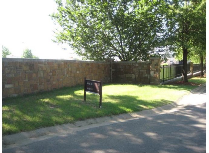
Figure 11: A2.2 to be repaired
