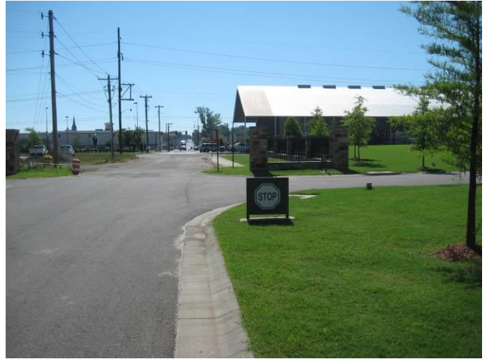
Figure 17: C1.6 to be repaired
