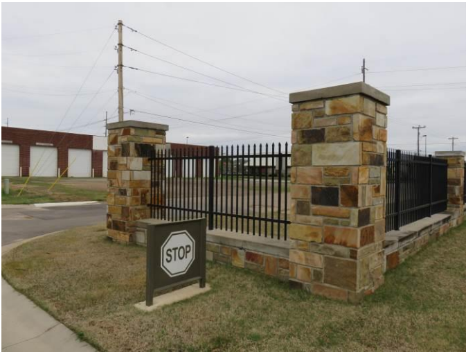
Figure 18: C1.7 to be repaired
