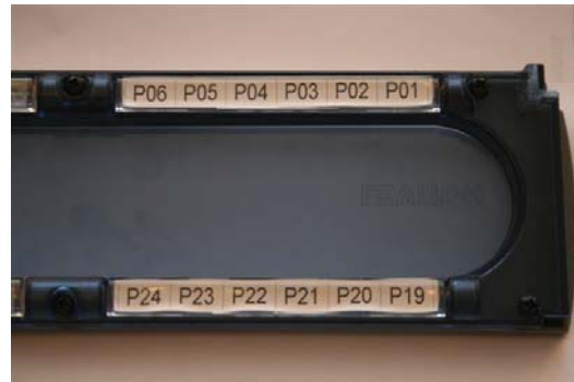
Inside Rear of Enclosure
