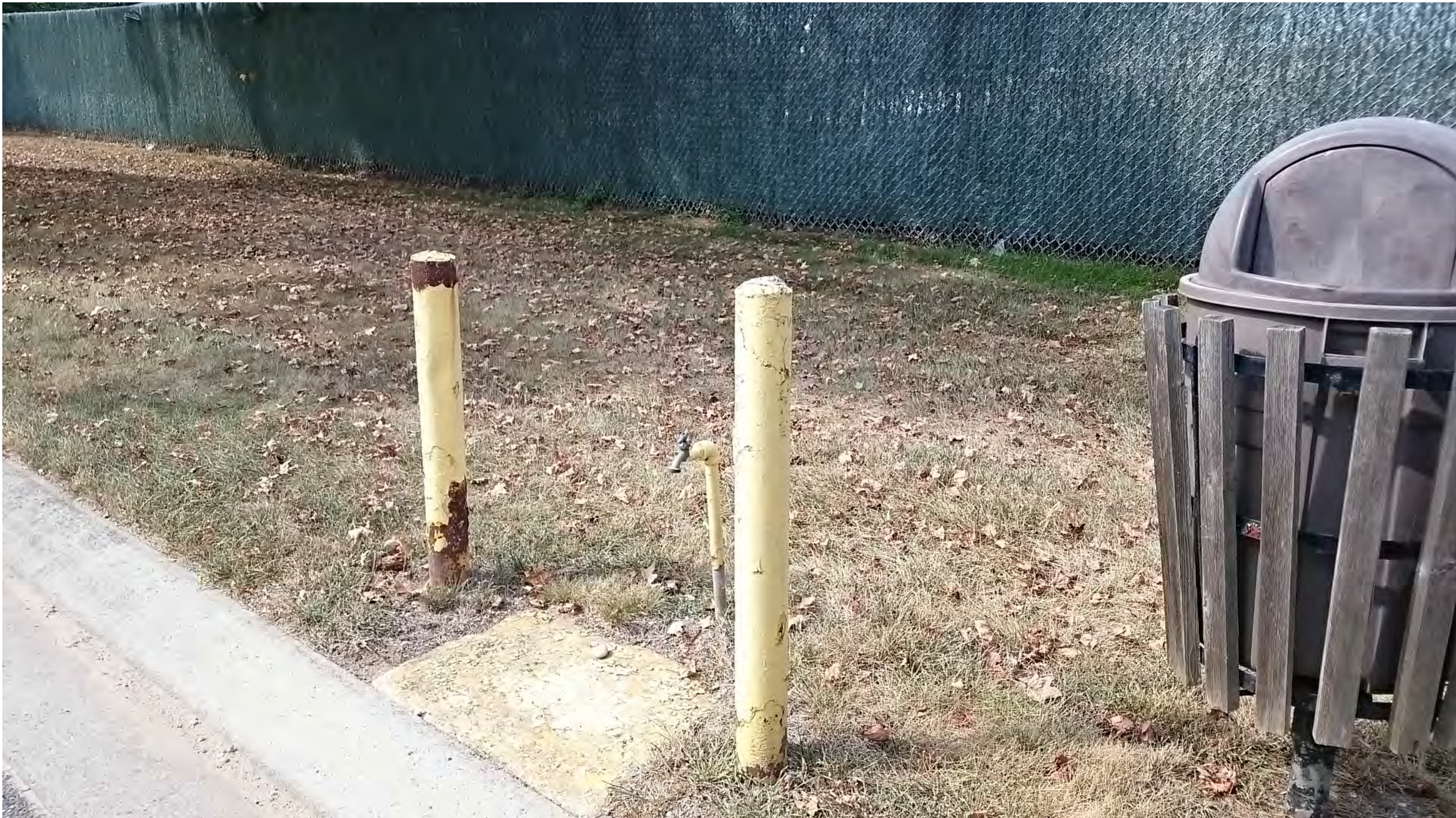
Detail 2: Picture showing the existing installations and conditions. Demolish all bollards, slabs, spigots, piping, trash cans, foundations, and structural supports either entirely or back to the specific point noted on other details and work descriptions.
