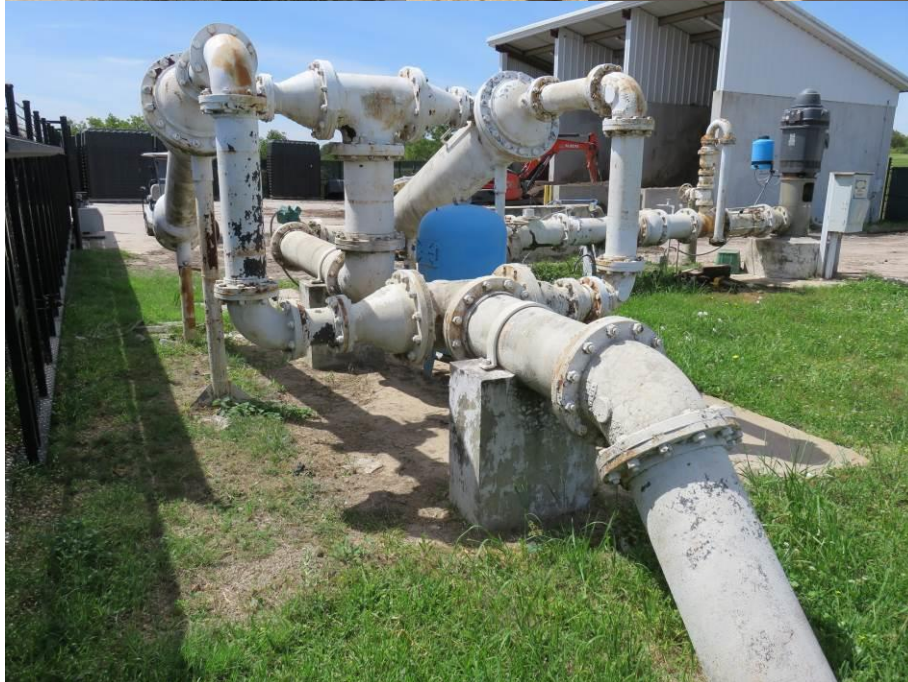
Figure 1: Eastern limits of work (blue expansion tank and circled sand separator not part of scope)
