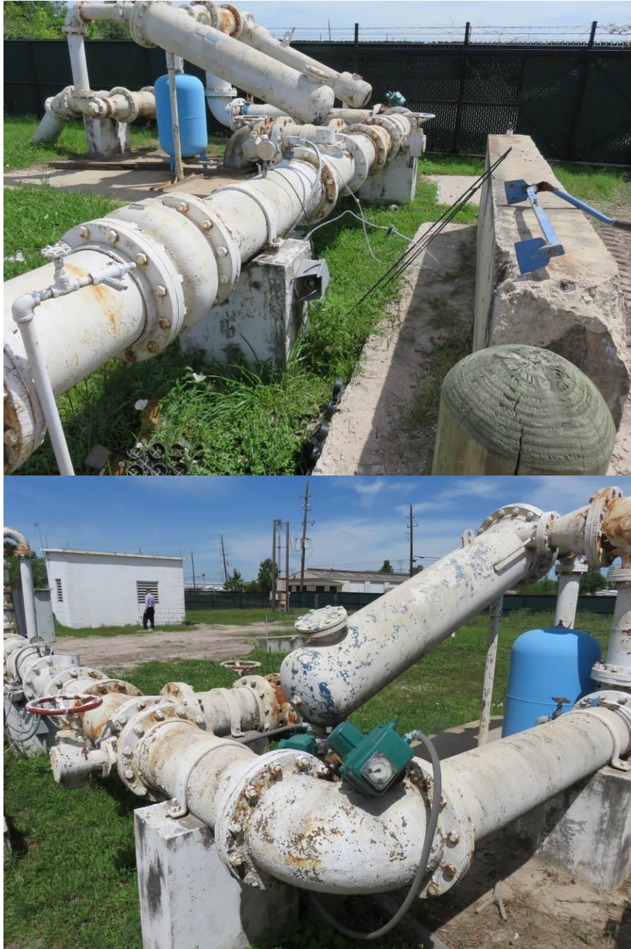
Figure 1: Opposite view of western limits of work Figure 2: Opposite view of eastern limits of work (circled sand separator not part of scope)
