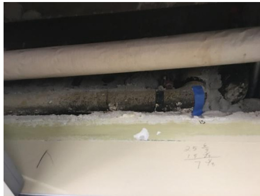
Asbestos Containing TSI- Sample 15
