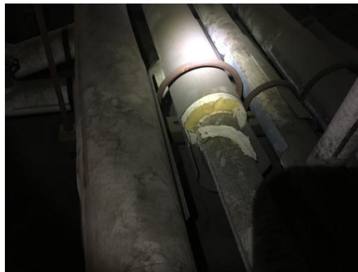
Non- ACM Insulation- Crawlspace
