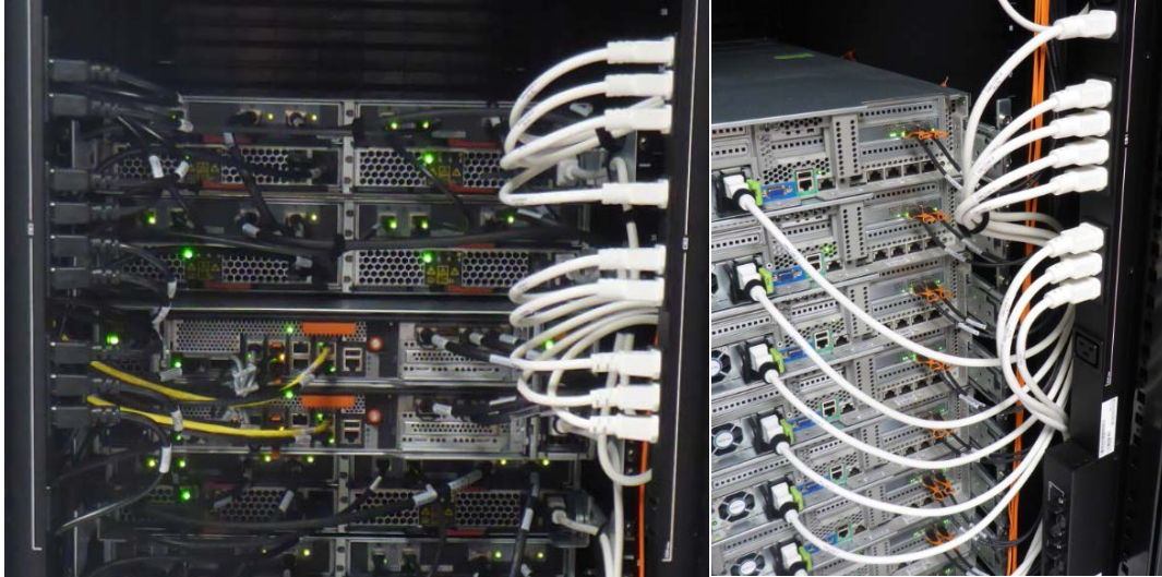
Figure 14: Example of Best-Practice Differentiated Power Cord Coloration Implementation
