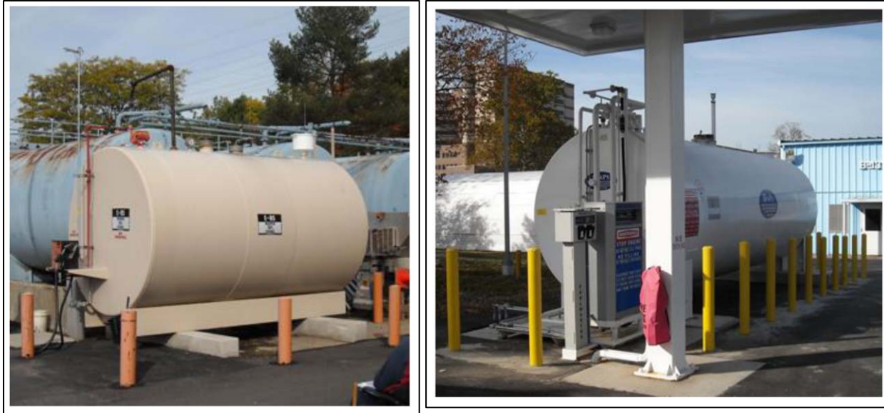
Figure 2-2. Examples of ASTs with E85 currently in use at VAMC campuses
